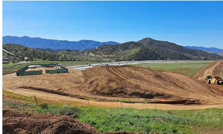
Storage area on the construction equipment pads alongside the dirt stockpile of +/- 120000 CY of dirt. (Installed bmp WM-1)
