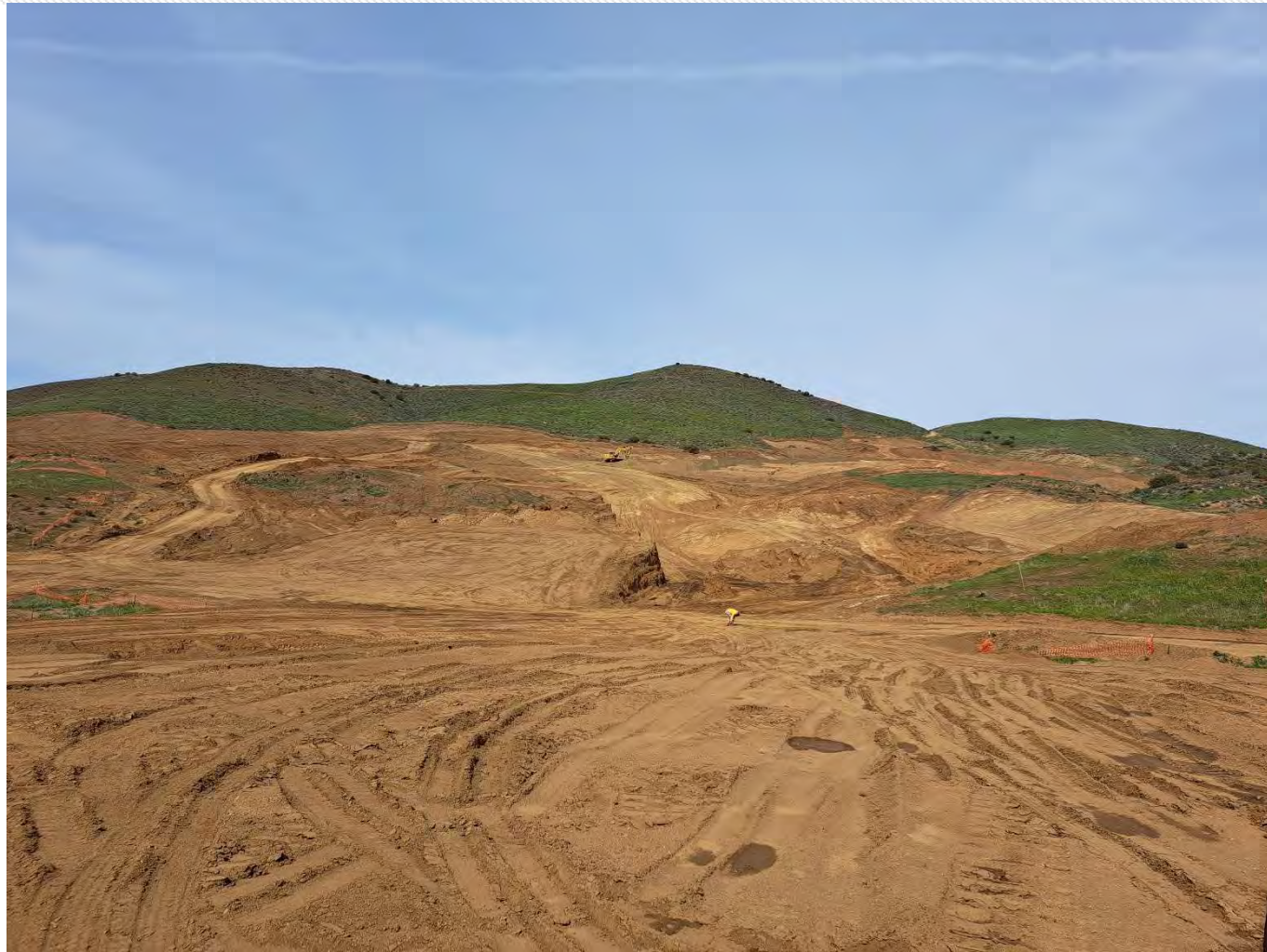
View of exposed bedrock along explored section of entrance access road from stockpile.
