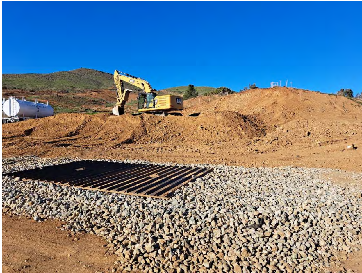
Picture taken during grading at the Valley Sage Entrance (10000 CY of the hill was cut and moved to stockpile).
