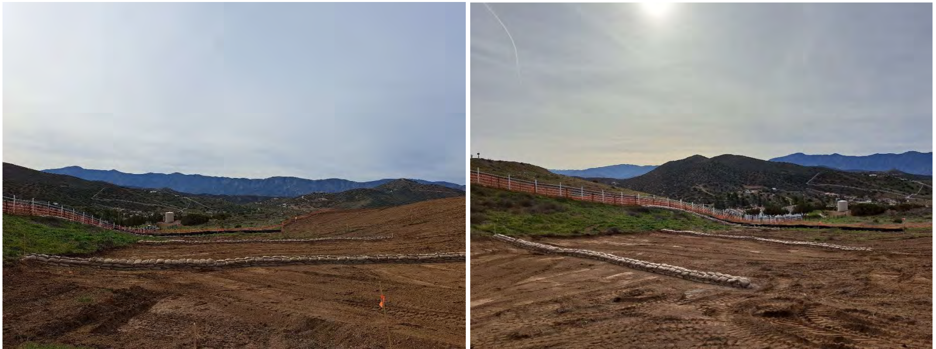
Check dams installed for erosion protection for the existing home(s) along the east side of TR 50381-01as per SE-4
