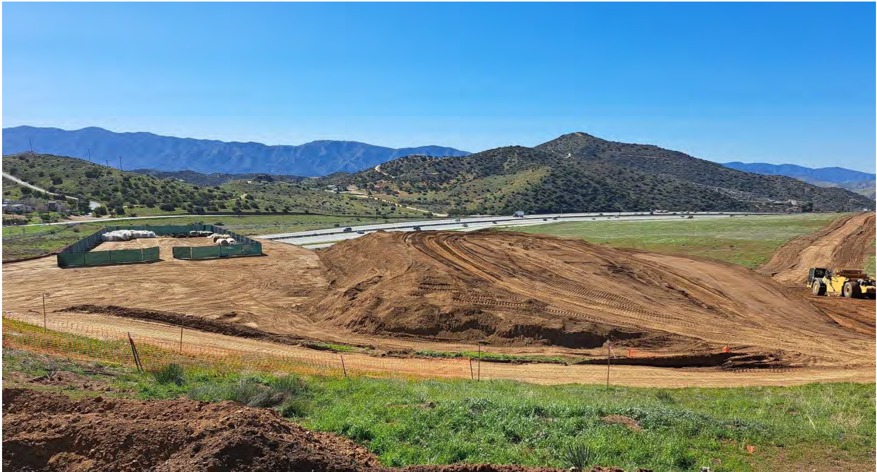
Storage area on the construction equipment pads alongside the dirt stockpile of +/- 120000 CY of dirt. (Installed bmp WM-1)
