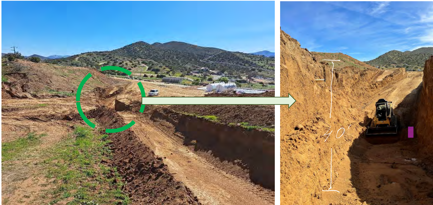
Exploration of bedrock along access road. Pictures facing from Valley Sage entrance along.
