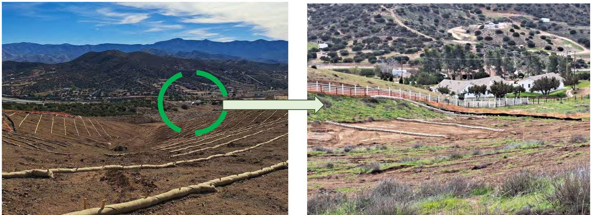
BMP's Installed as per approved winterization plan, using sandbags, silt fence and wattles on the eastern end of the property close to Mr. Estes's residence.
