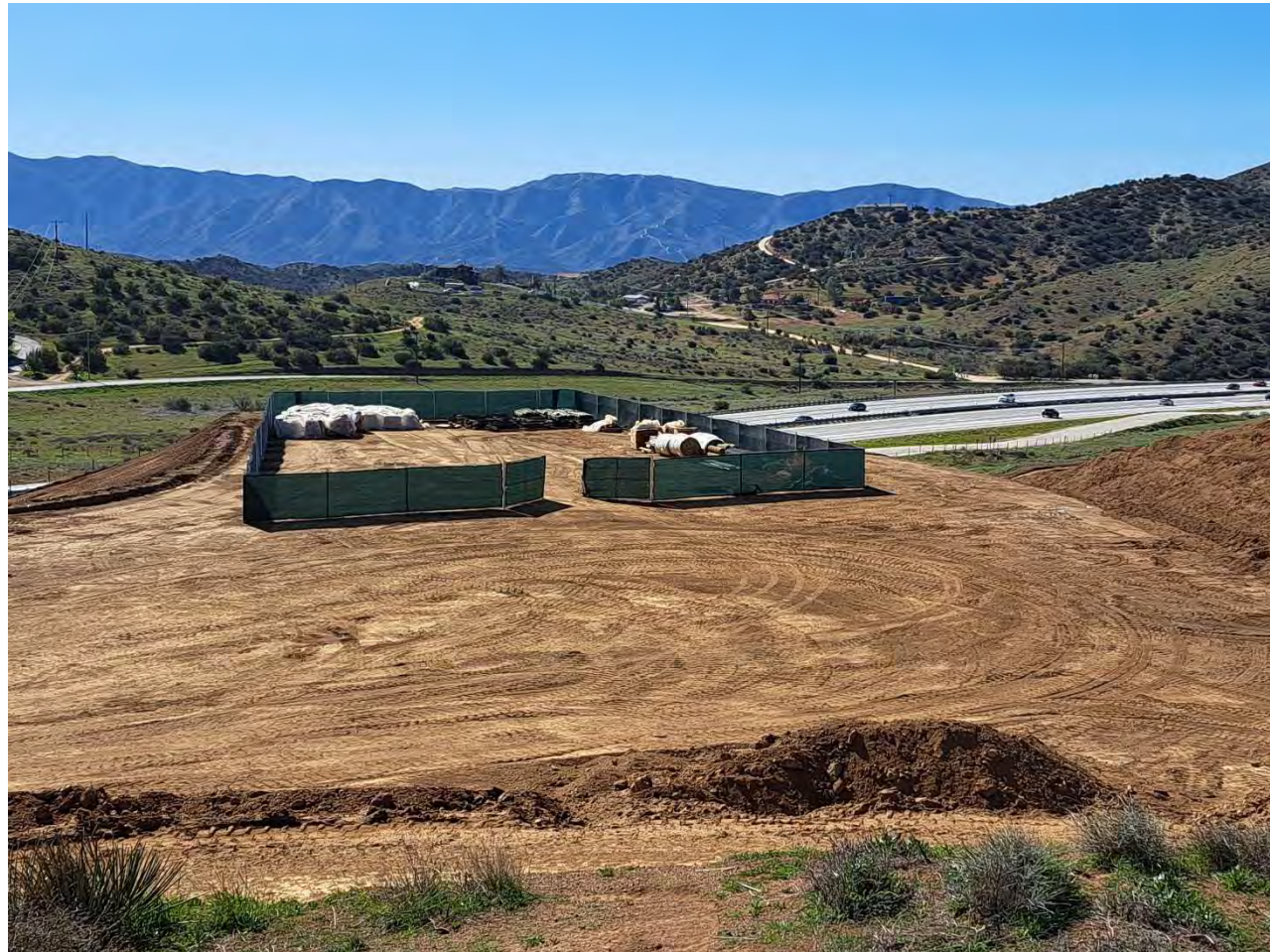
Completed reconstruction of chainlink fence for equipment yard / storage area. (Installed bmp WM-1)
