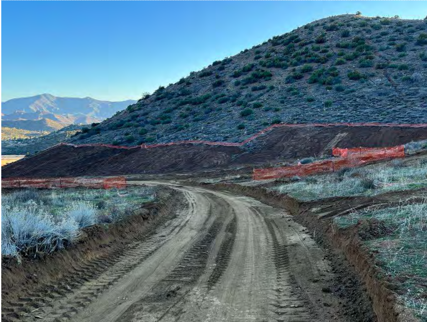
Pictures showing brush cleared area on the SW part of the site.
