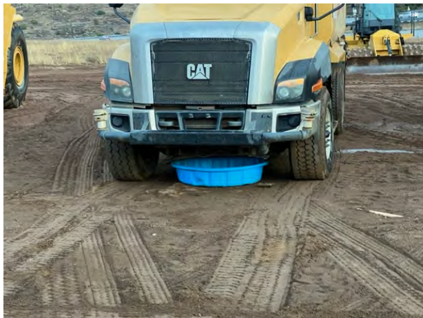
Drip pans for spill prevention and control (WM-4)
